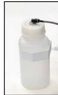
Fig. 5: Check of condensate collection vessel
