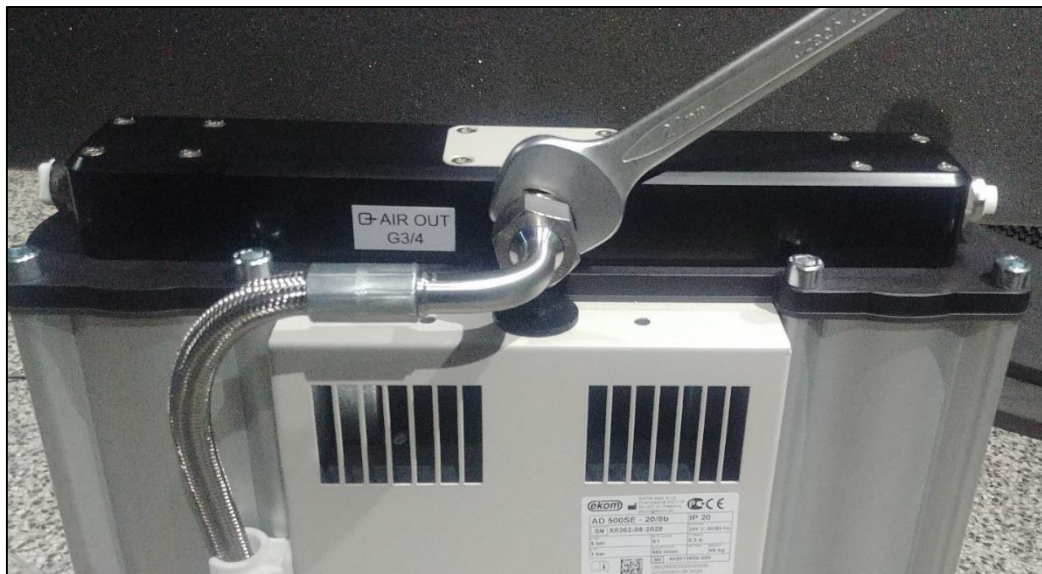
Fig. 10: Compressed air outlet
