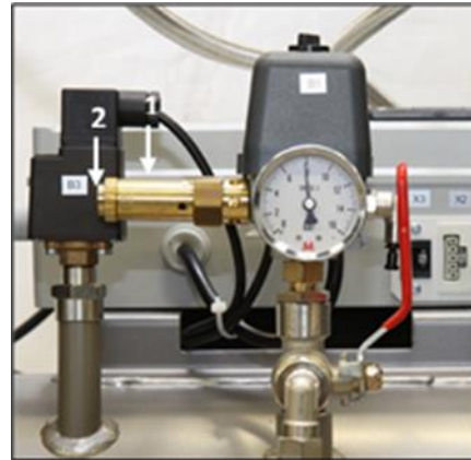
Fig. 22: Check of safety valve
